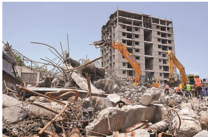
Fig -1: Construction Waste
