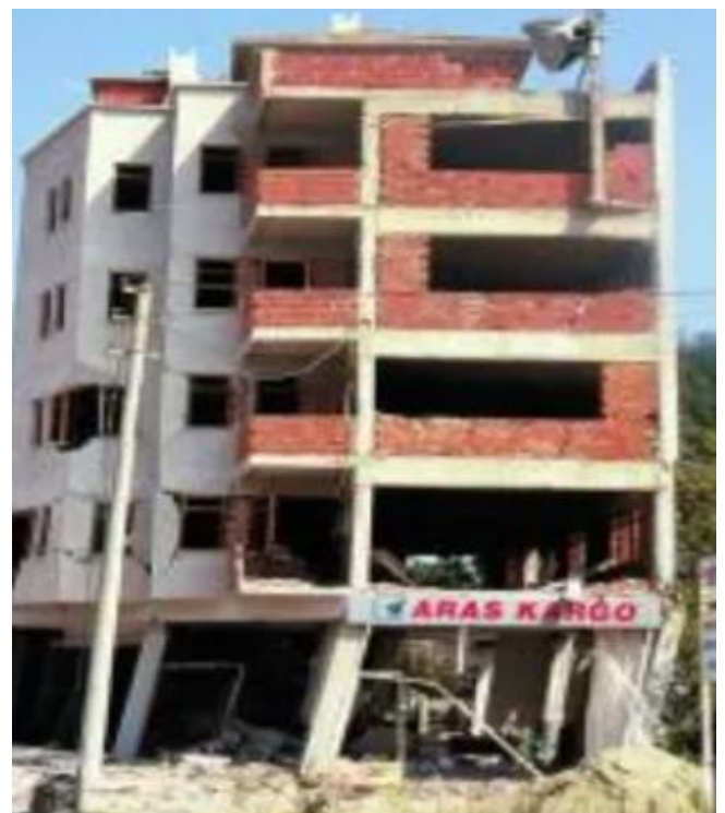
Fig. 2 Failure of stilt floor during earthquakes
