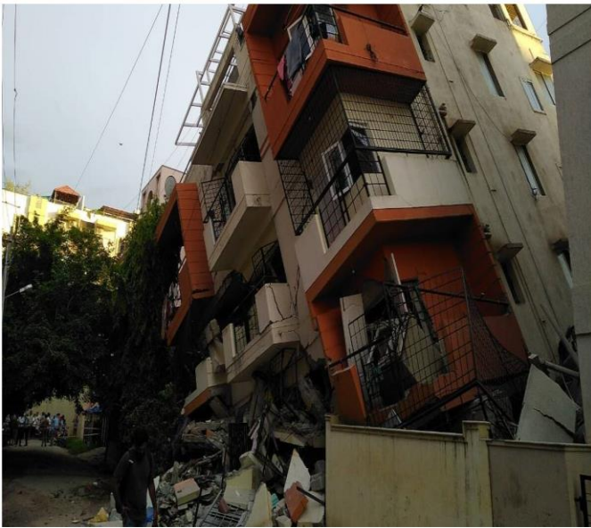
Fig. 6 collapse of apartment building Bangalore.
