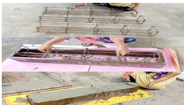
Fig.6. Placing of reinforcement in the beam moulds & Finishing of RCC beams after casting
