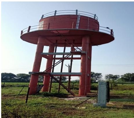
Fig -1: Elevated storage tank
