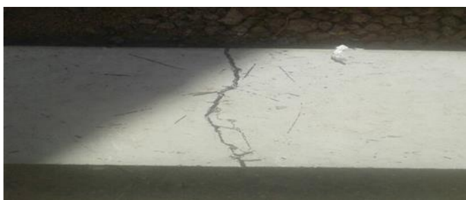
Fig. 13: Ultimate failure for 1.0 % PFRC beam
