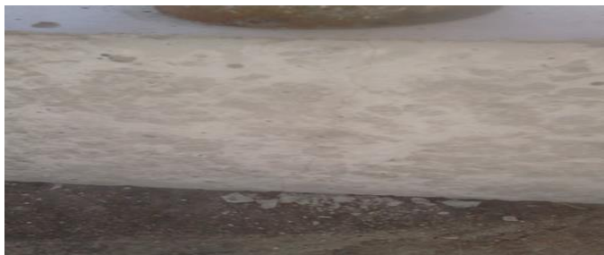
Fig. 12: First crack appearance for 1.0 % PFRC beam
