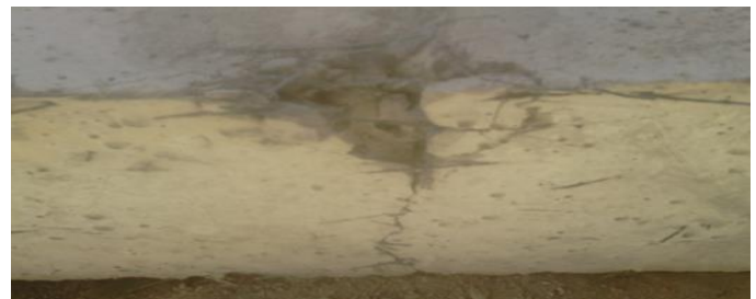
Fig. 15: Ultimate failure for 2.0 % PFRC beam
