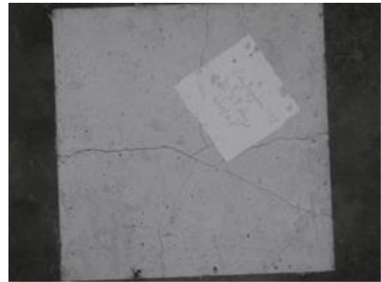
Fig. 9: Cracks for polypropylene fibre slab
