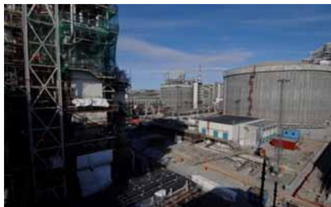
Plate 1: Typical Process Facility and Storage Tanks [5].
