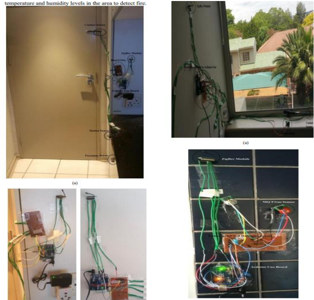
temperature and humidity levels in the area to detect fire.
