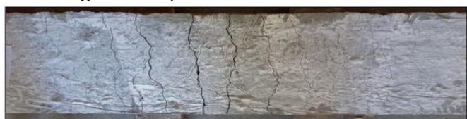
Fig. 6: Crack patterns of HFRP slabs
