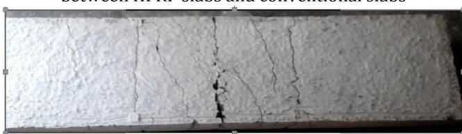
Fig. 5: Crack patterns of conventional slabs
