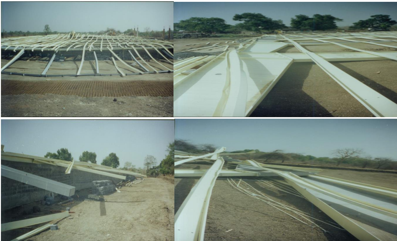
Fig.1 Pack of Cards Failure – Building Collapsed In Direction of Ridge.
