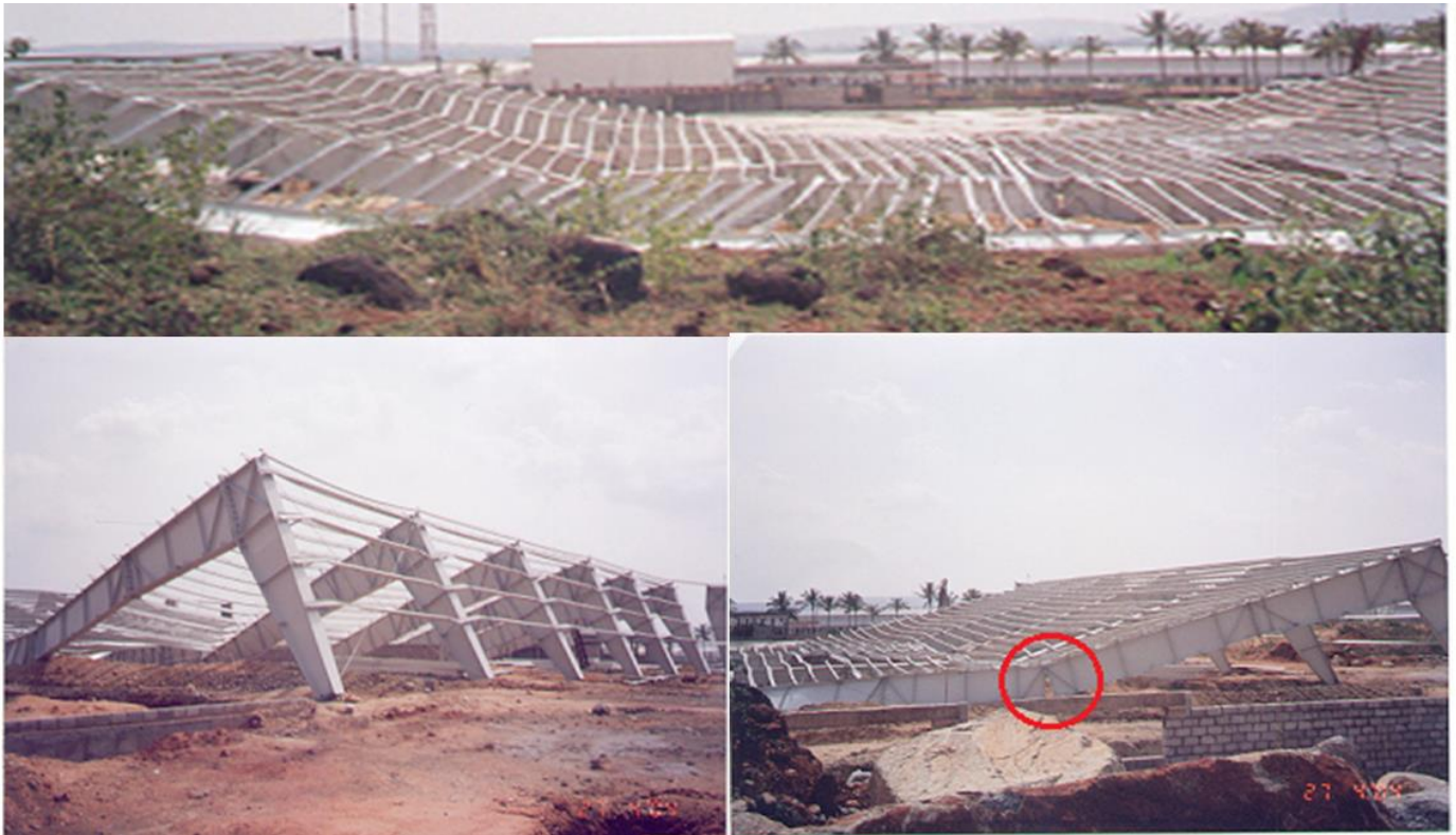
Fig. 2. Failure in Plane of Due to Rafter Splice
