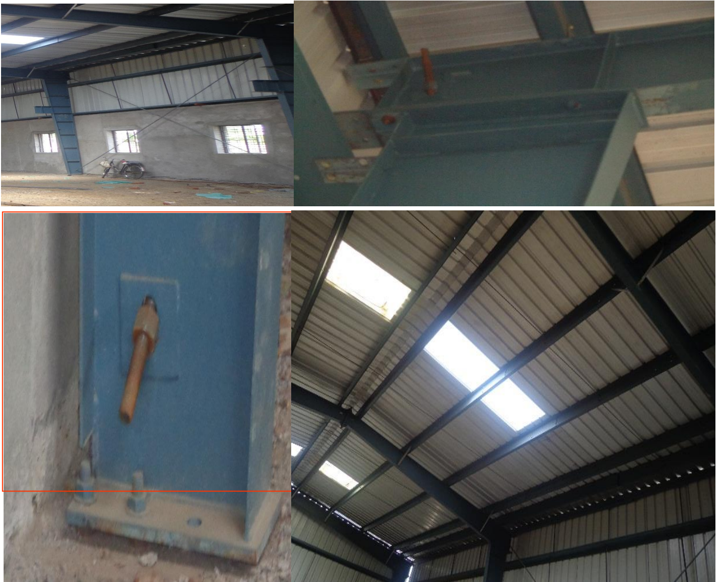
Fig. 15 Outer Flange Cut, Mismatch in Knee Splice Plate, Wrong Bracing and Midspan Purlin Laps
