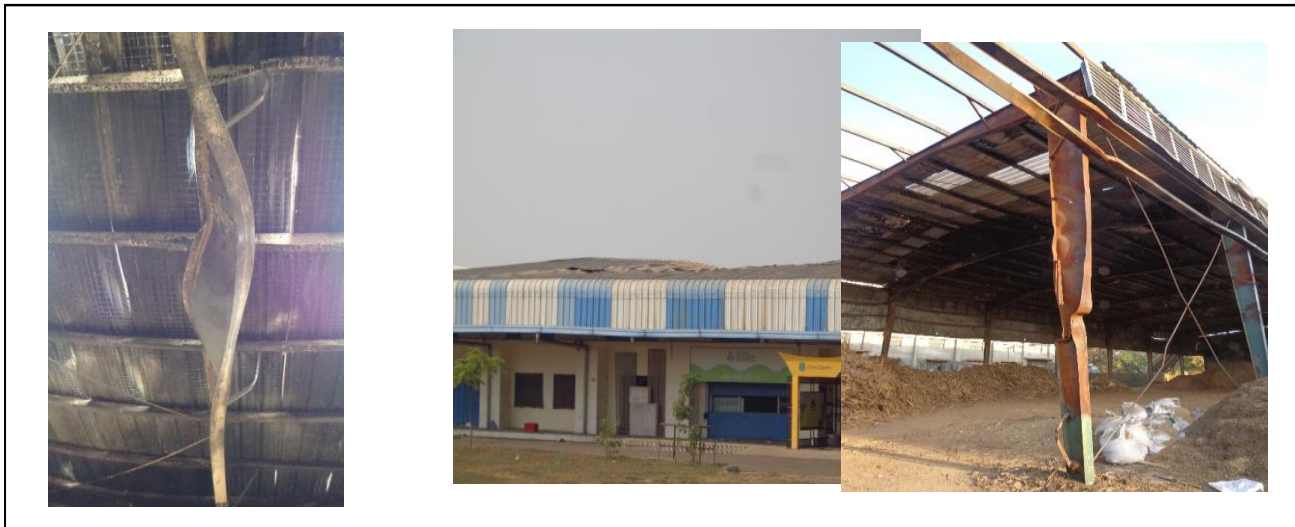
Fig. 10 Building Collapse – Partial and Complete Due to Fire Accidents, Sagging Roof
