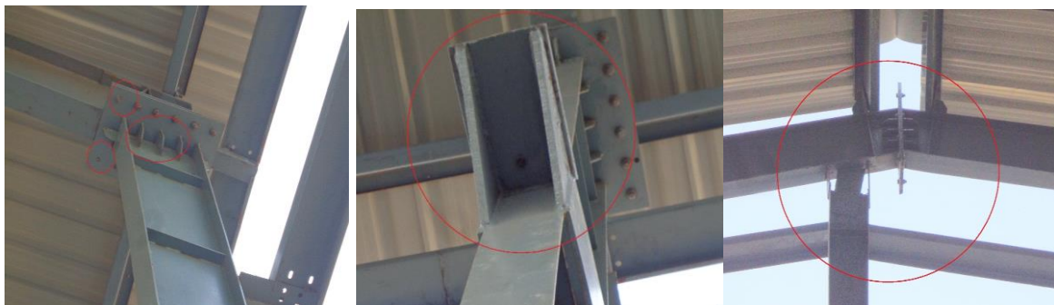
Figure 12 Poor Splice, Crane Bracket Detail and Endwall Column Top Splice with Rafter
