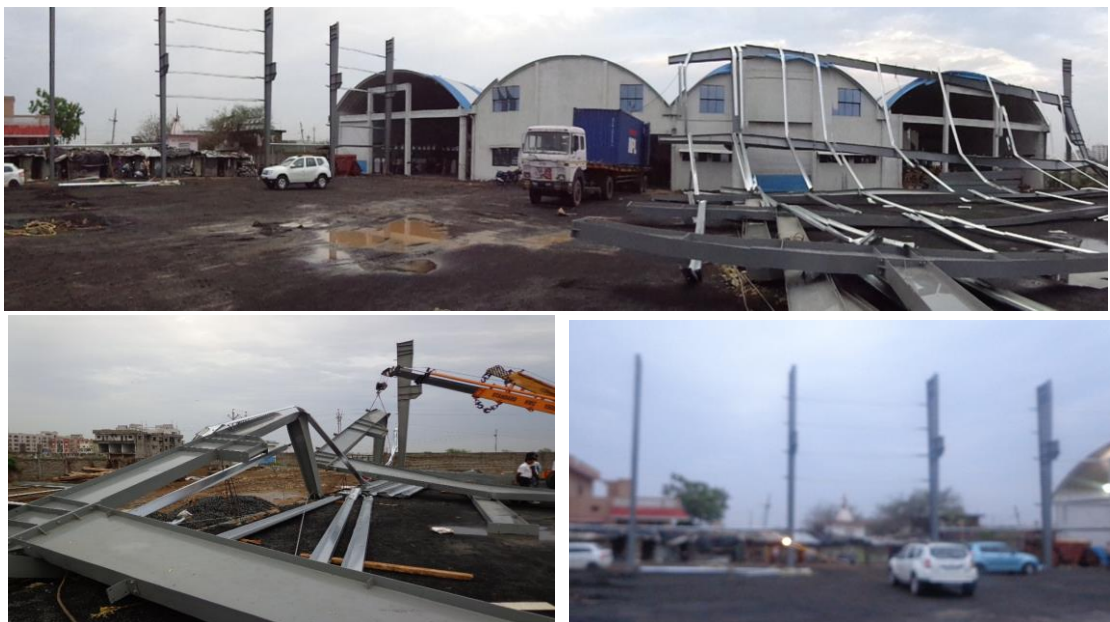
Fig. 3. Building Collapse along Ridge and Unbraced Free Standing Columns
