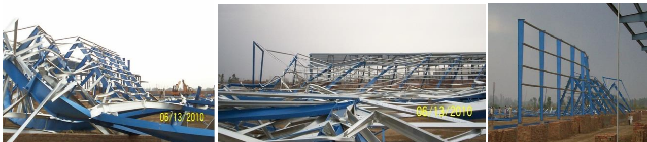
Fig. 9 Collapse of a Building in Plane of Frame and Unbraced Free Standing Columns
