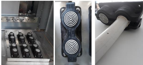
Fig -29: Cable lead-throughs (Fimer: PVS 980 inverter)
