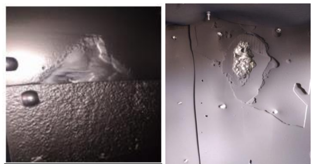
Worn cabin NI hard liner
