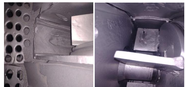
Wear of Straight liner
