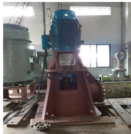
a) Front view of testing arrangement of pump
