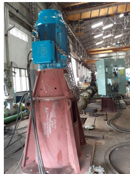
b) Side view of testing arrangement of Pump
