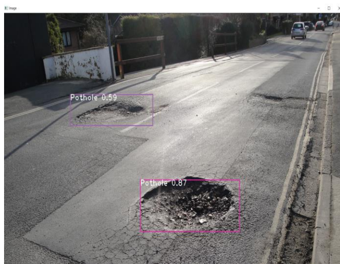
Fig3. Pothole detected by custom trained EfficientDet
