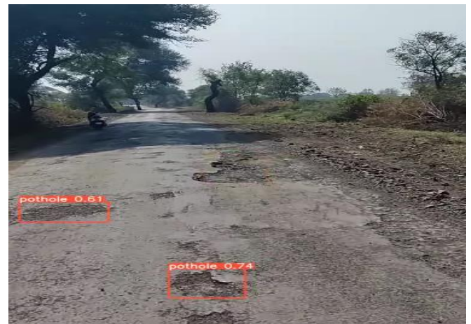
Fig4. Pothole detected by custom trained YOLOV5
