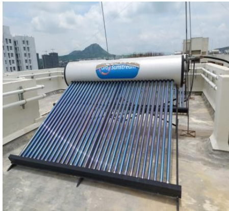
Fig-7: Solar powered water heater
