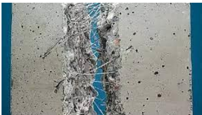
Fig 2.1 Cracking of Non- Reinforced Concrete
