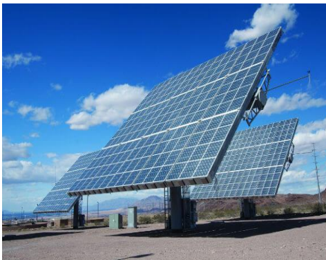
Fig -7: Concentration PV module
