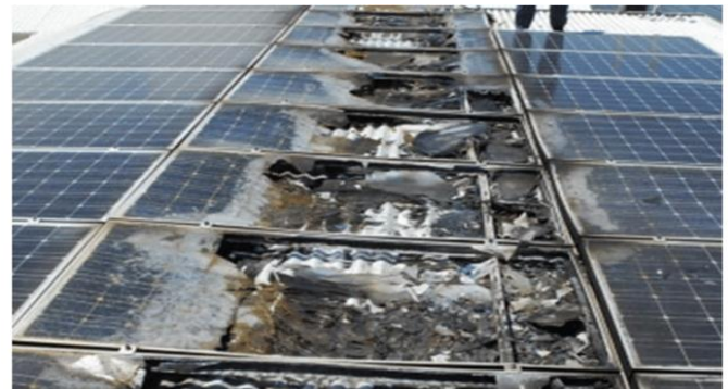
Fig. 1: Damage to a PV system attributed to an arc
